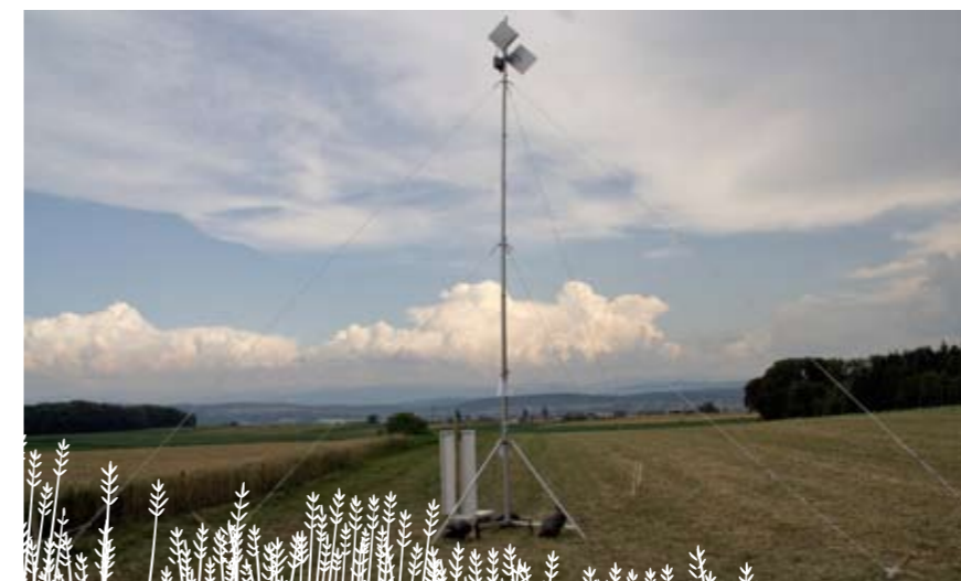
Solar-powered mesh node with directional antennas.
